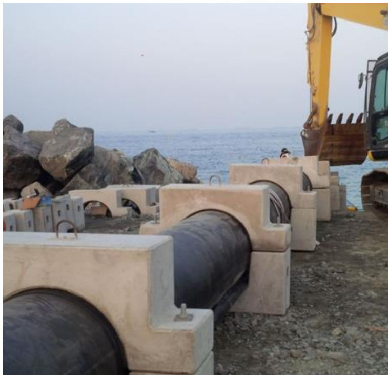
Photo 7-1. Subsea pipe string assembled in an onshore stringing yard, fitted with concrete weight collars.
