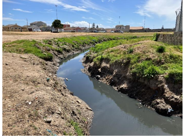
Photo 2-10. Open stormwater channel downstream of Milky Way culverts – this water passes out via the Erica Road culvert downstream
