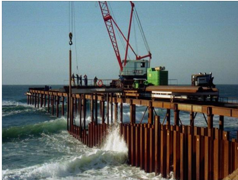
Photo 7-2. An example of construction of a sheet-piled cofferdam to protect the excavation of a pre-trenched shore crossing.
