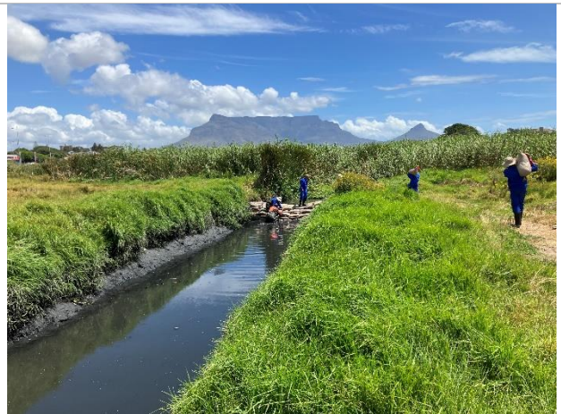
Photo 2-12. Erica Road culvert showing sand bags to assist in over-pumping to the adjacent sewer
