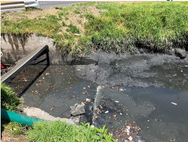
Photo 2-11. Polluted stormwater lowflows are pumped out of the open outfall at the Erica Road culvert and discharged into the adjacent sewer manhole
