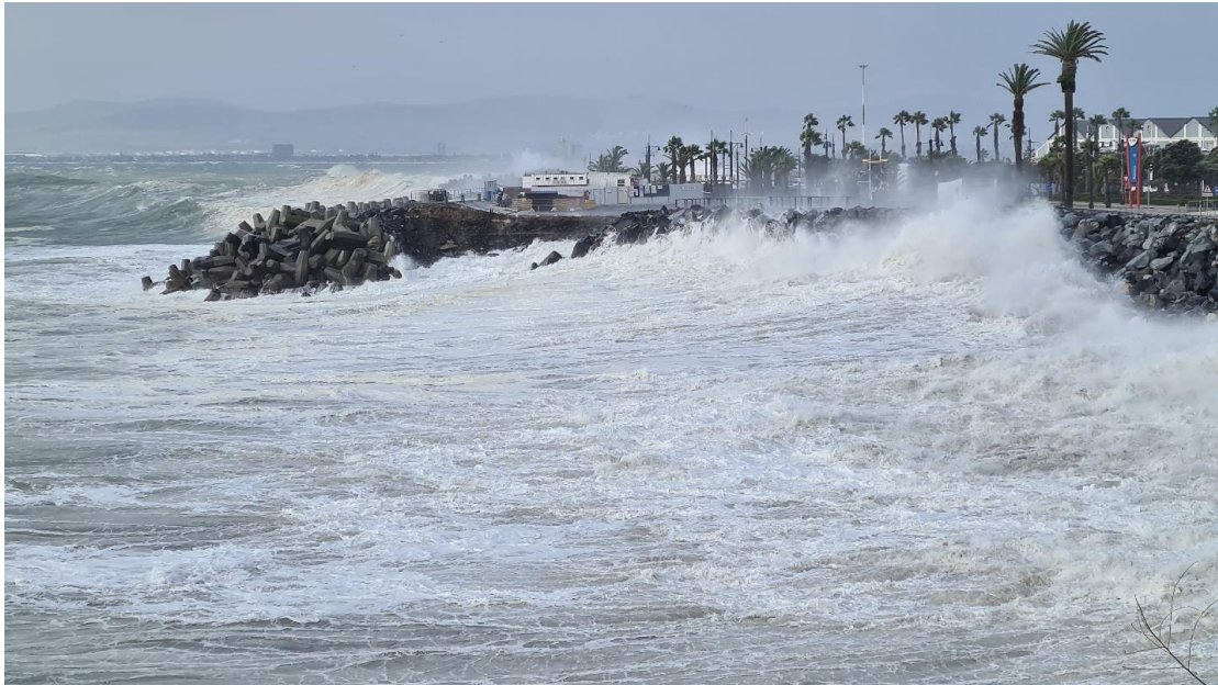
Figure 2-17: Overtopping of rock revetment at approximately 15:00 on 13 July 2020. Photo credit: Stephen Luger.
