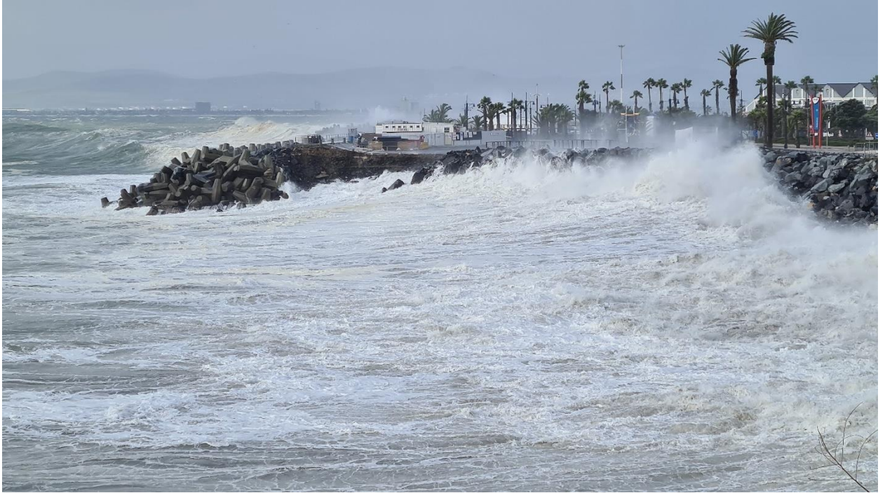
Figure 5-9: Overtopping of rock revetment at approximately 15:00 on 13 July 2020. Photo credit: Stephen Luger.
